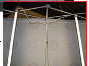
Link cable connection close up.
